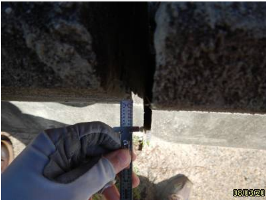
Photo 4 – Horizontal Misalignment at Bent 13
