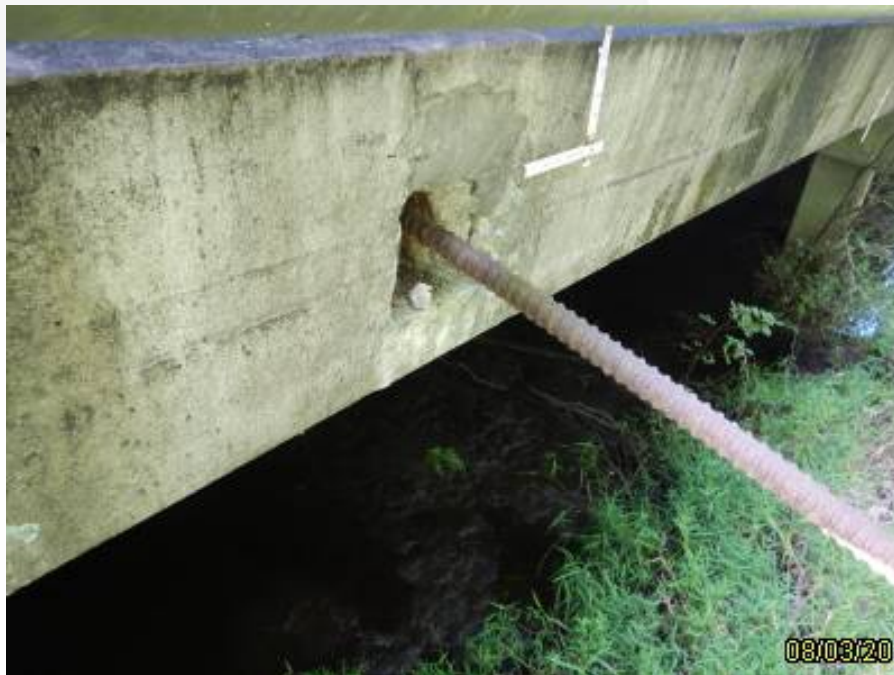
Photo 2 – Broken Post Tensioning Bar in Span 22
