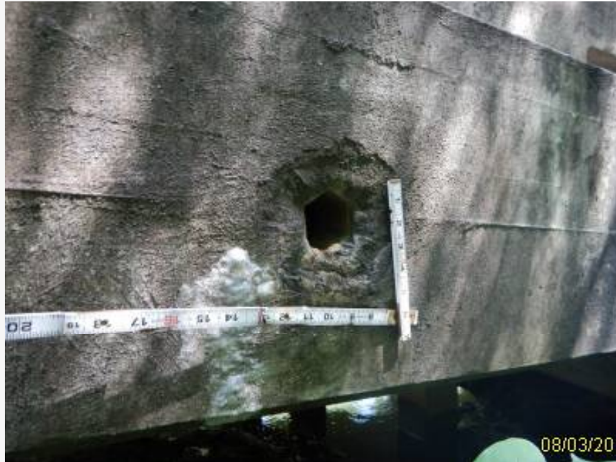
Photo 1 – Missing Post Tensioning Bar in Span 5
