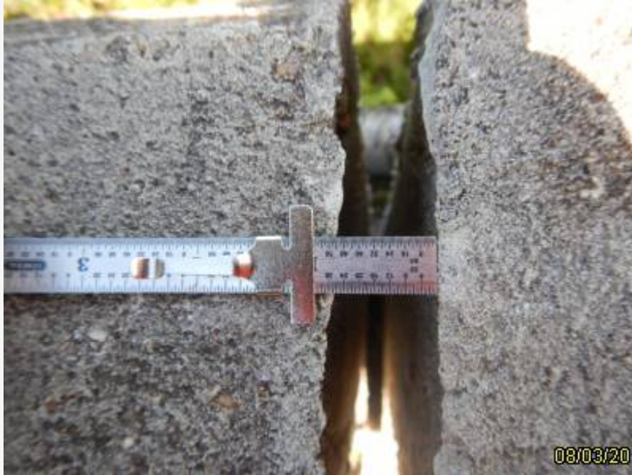
Photo 3 – Bridge Rail Offset at Bent 8
