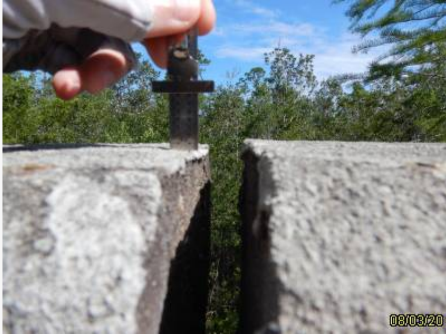
Photo 5 – Bridge Rail Vertical Alignment at Bent 43
